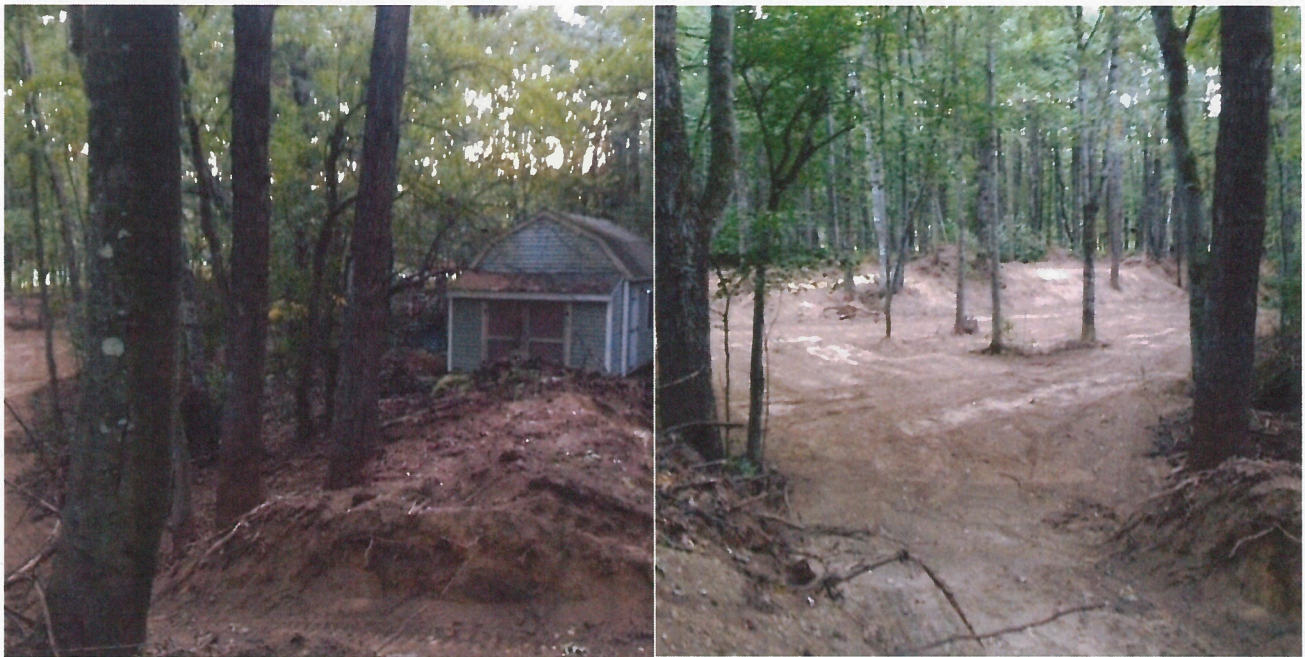
Depressional Areas during unpermitted excavation 2016
