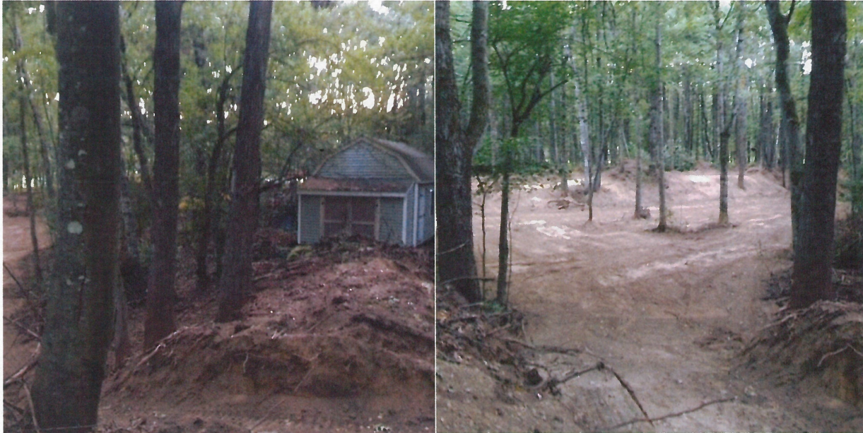
Depressional Areas during unpermitted excavation 2016
