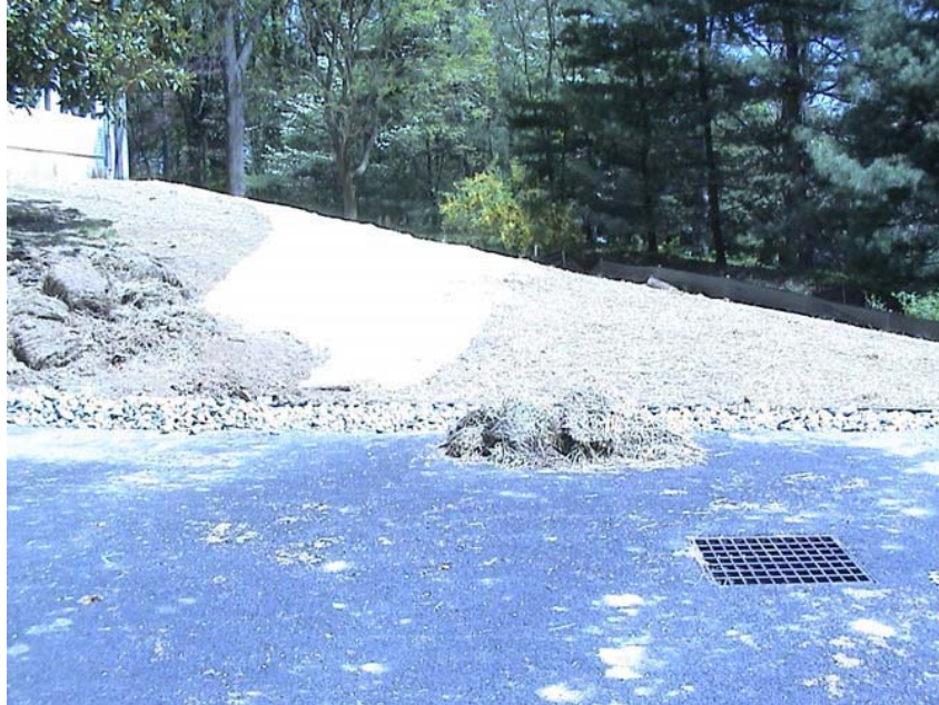
Figure 2: Example of soil wash-on/dumping from unstabilized landscaping.
