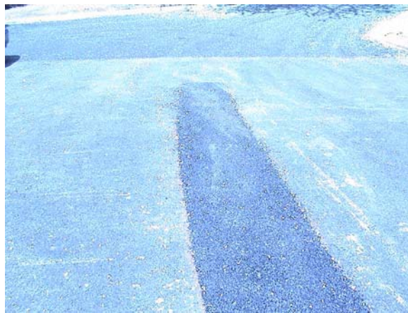
Figure 6: Standard bituminous patch in porous asphalt parking lot. This lot was constructed with an unmodified porous mix (i.e. no polymer modification) and had rutted in the center of the aisle due to construction traffic.
