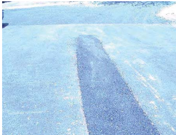
Figure 6: Standard bituminous patch in porous asphalt parking lot. This lot was constructed with an unmodified porous mix (i.e. no polymer modification) and had rutted in the center of the aisle due to construction traffic.
