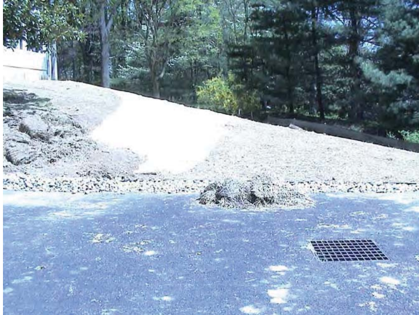
Figure 2: Example of soil wash-on/dumping from unstabilized landscaping.
